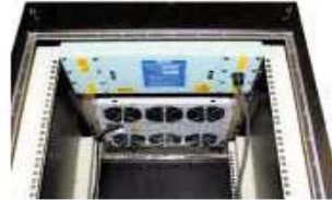
Inside I/O panel + fans
